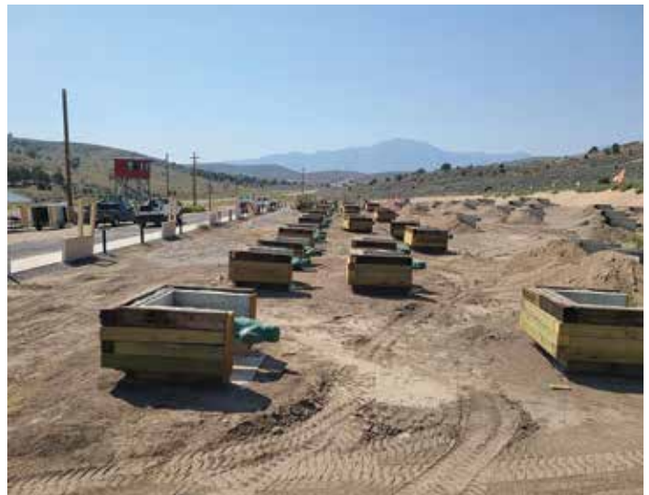
In September of 2021, the Combat Pistol Range underwent upgrades conducted by Range Control's downrange maintenance crew to improve safety, in accordance with the new pistol qualification standards. This enhances use of the range by service members and local law enforcement.
