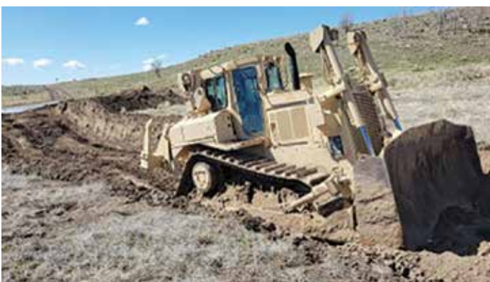
A Soldier from the 116th Engineer Company operates a D-7 bulldozer in performing a horizontal construction mission on Camp Williams, Utah, during annual training in May 2021.
